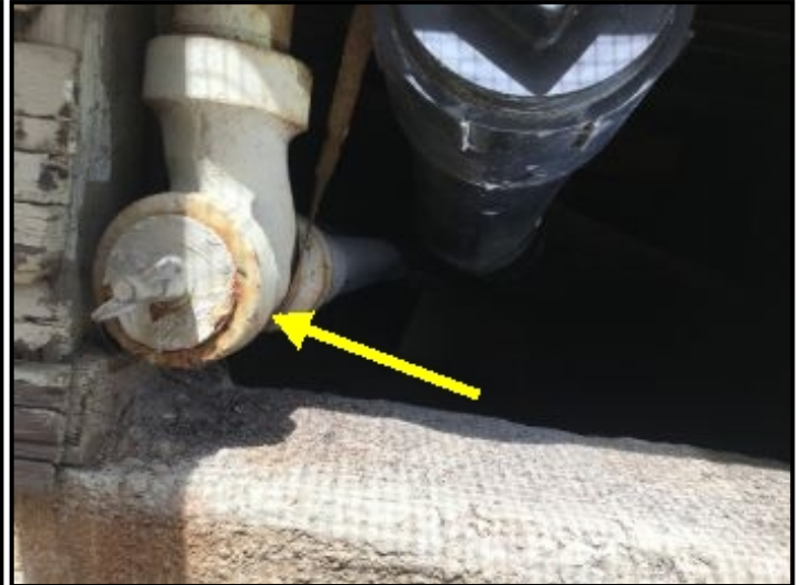
cast iron drain clean out
