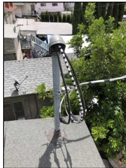
overhead service mast
