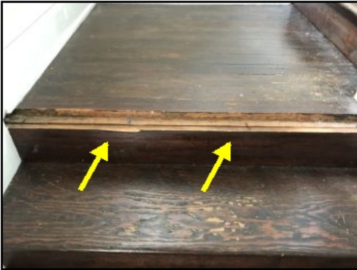
damaged stair at landing
