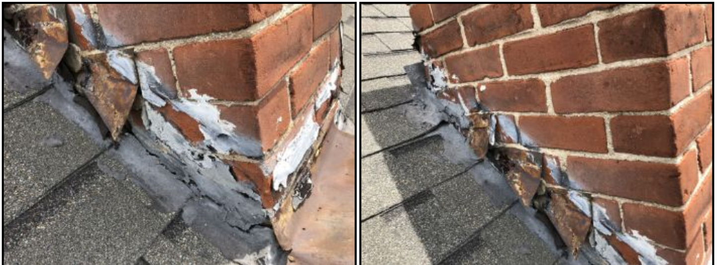
damaged chimney flashing
