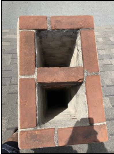
No liner - no cap /spark arrestor
