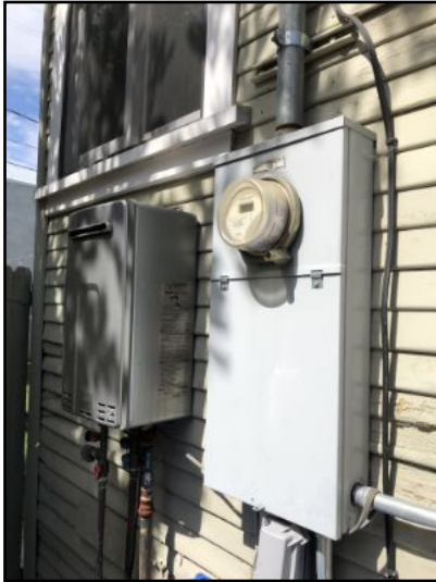
meter and panel
