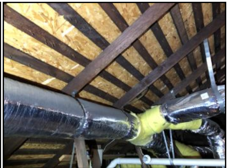
HVAC duct work
