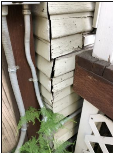
Deterioration of wood siding
