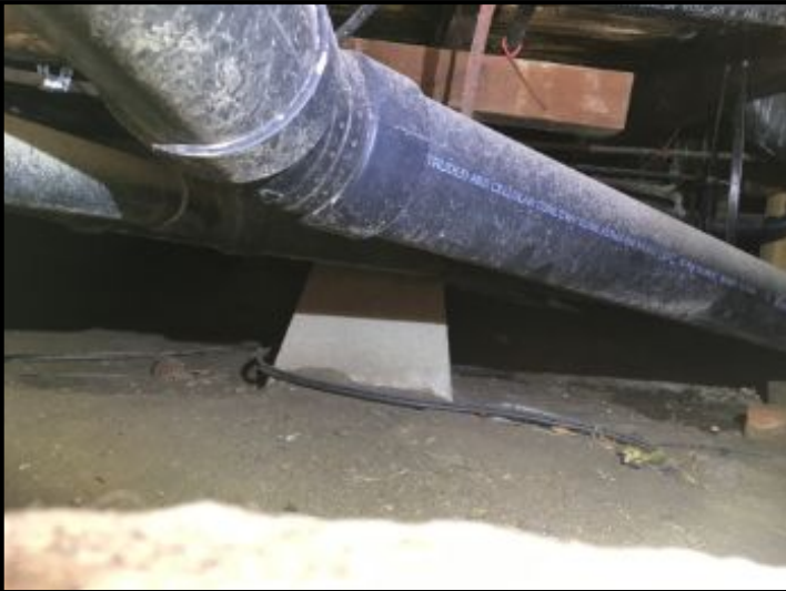
ABS drain lines present
