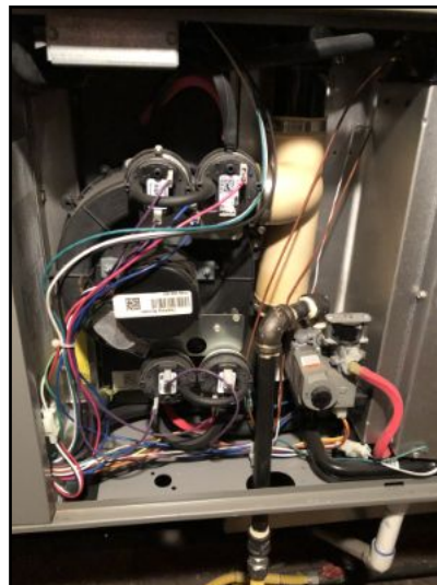
burner compartment clean
