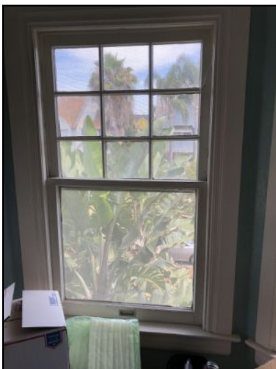
balance broken at older window
