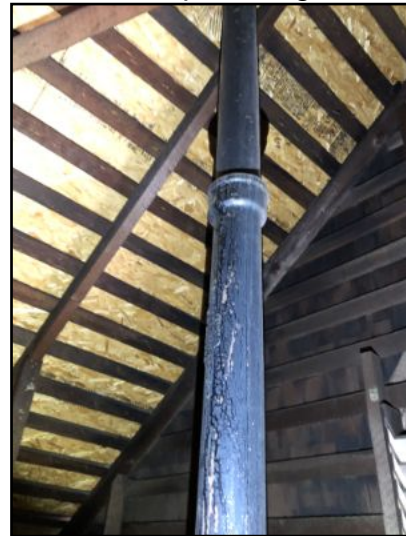
Cast iron vent stack
