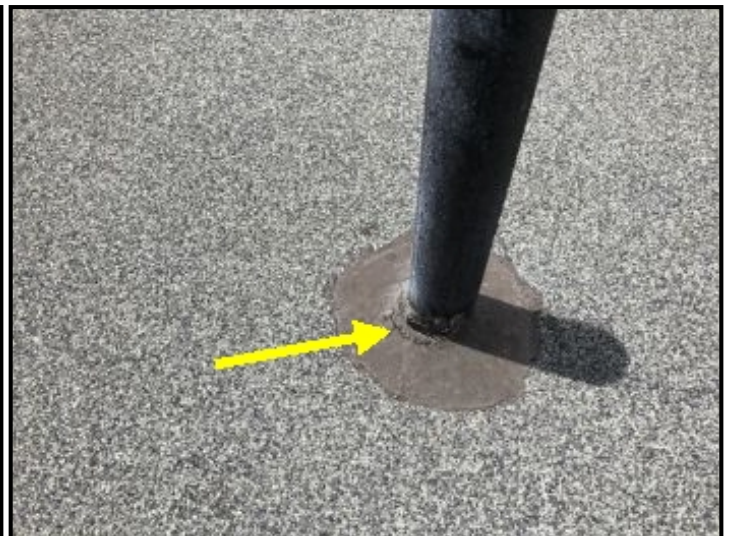
No flashing at PVC vent stack
