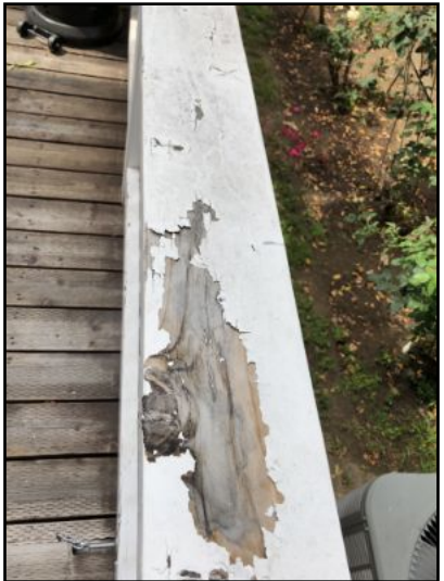
paint needed at railing
