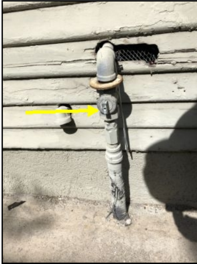
main gas shut off
