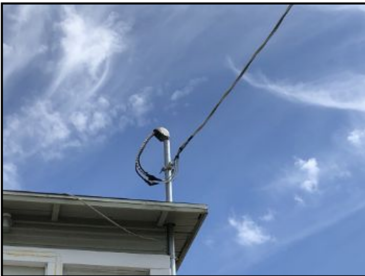
overhead service mast
