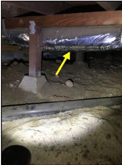
HVAC flexible duct work found
