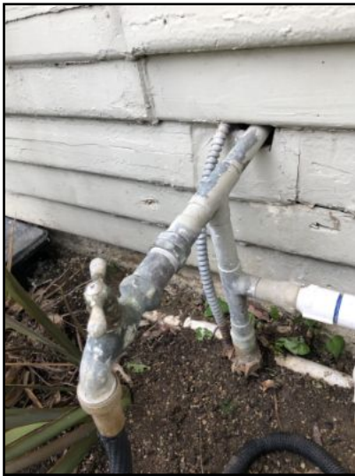
No anti-siphon device
