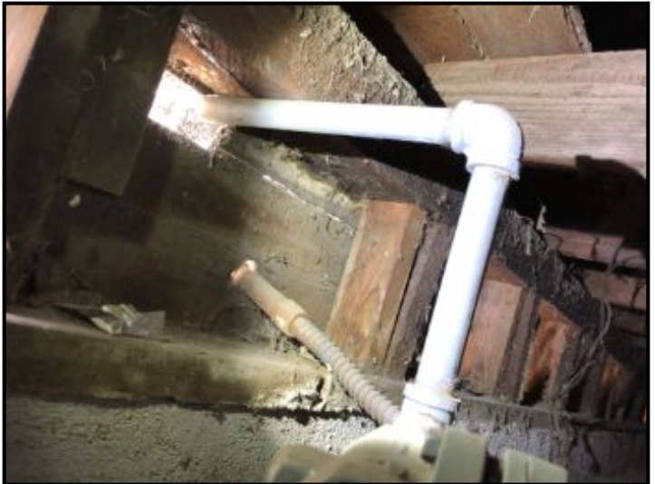
no plywood added on eastern wall in crawlspace
