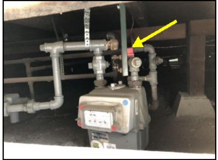
gas meter - note seismic auto shut off valve
