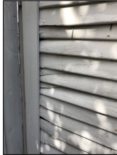
deterioration of wood siding
