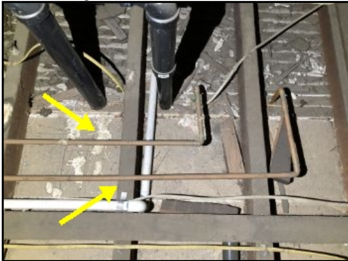
copper water supply lines
