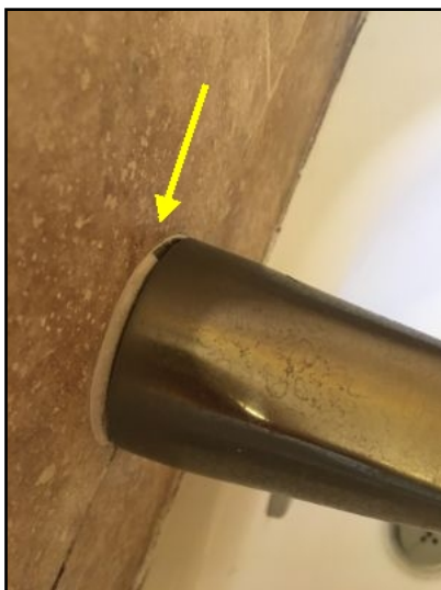
gap at tub faucet
