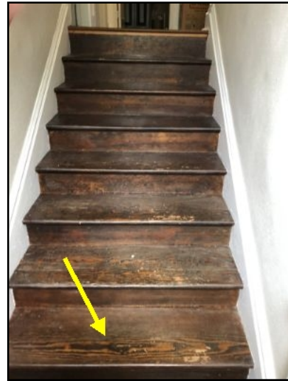
damaged bottom step
