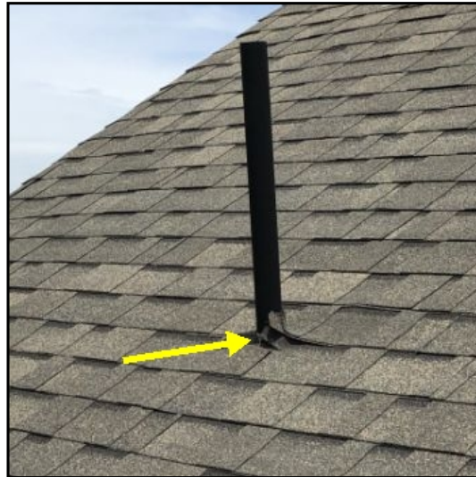
No flashing at ABS vent stack
