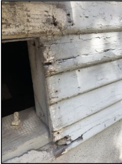
wood siding deterioration
