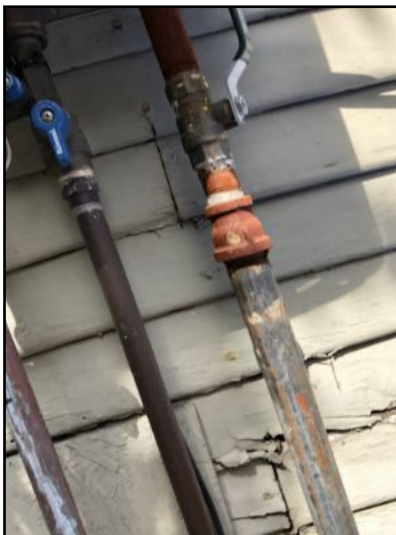
gas shut off for tankless water heater - no sediment trap
