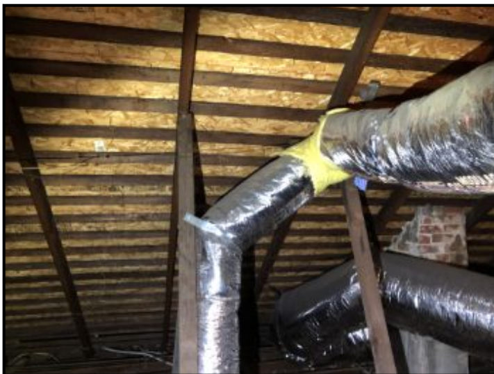
HVAC duct work
