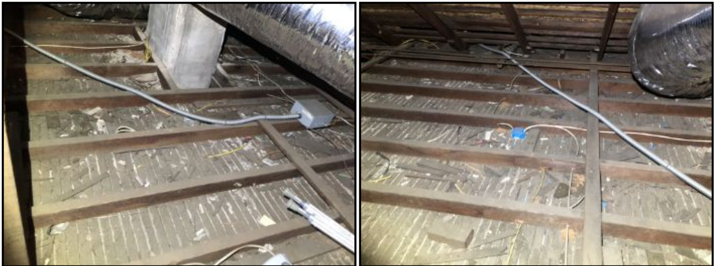
no insulation on attic floor
