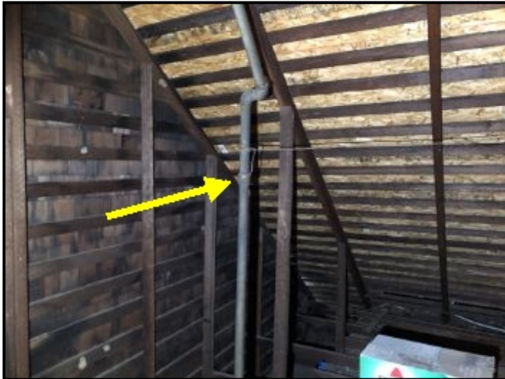
galvanized steel vent stack
