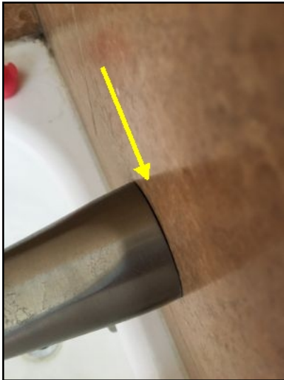
gap at faucet
