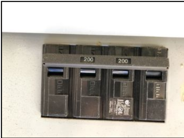
200 AMP main breaker
